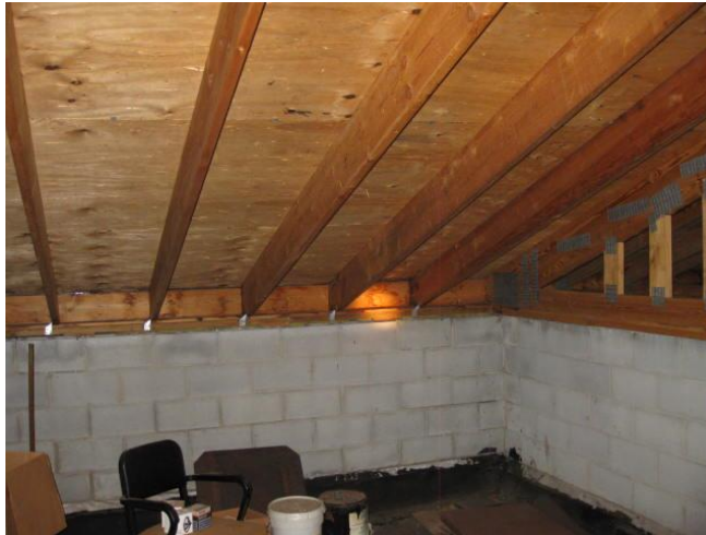
Photo 2 – truss blocking ventilation at exterior wall
