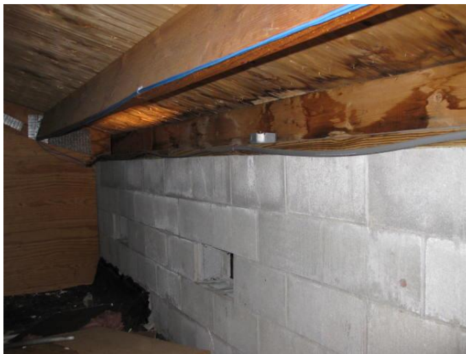
Photo 3 – rafter blocking ventilation at exterior wall
